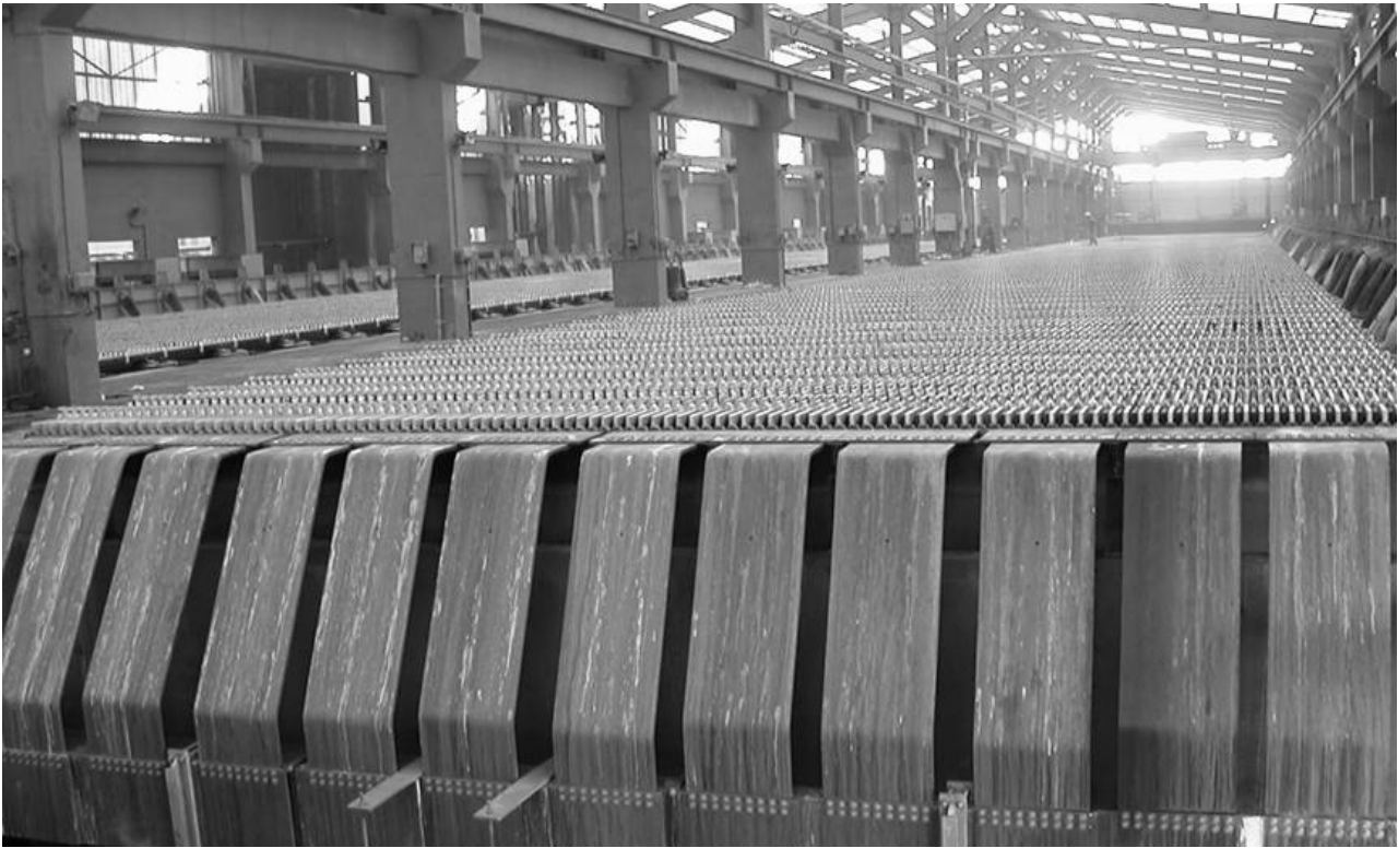
Figure: 12 riser bars feeding the end cell with a current of approx. 200 kA which leads to a nominal current of 16,5 kA per riser bar.
